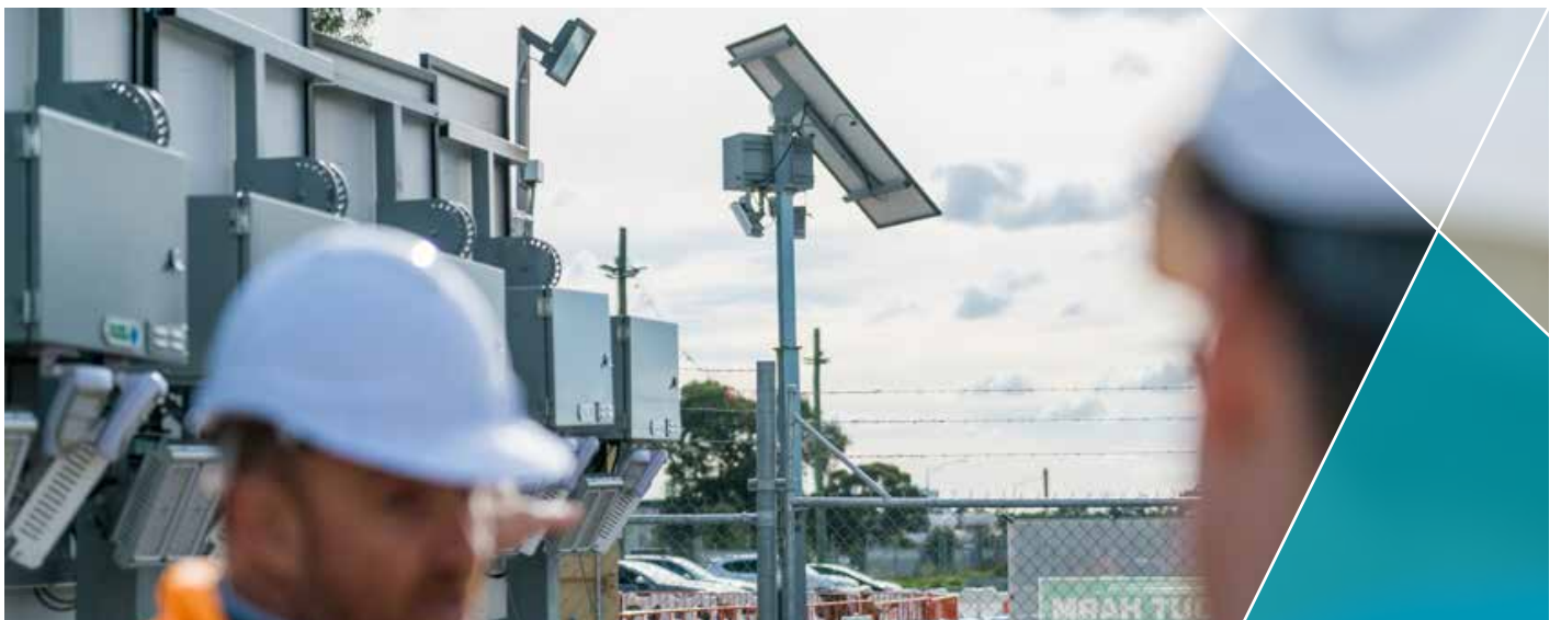
Solar powered light stands
